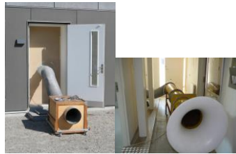
Figure 3. Fan and venturi setup
